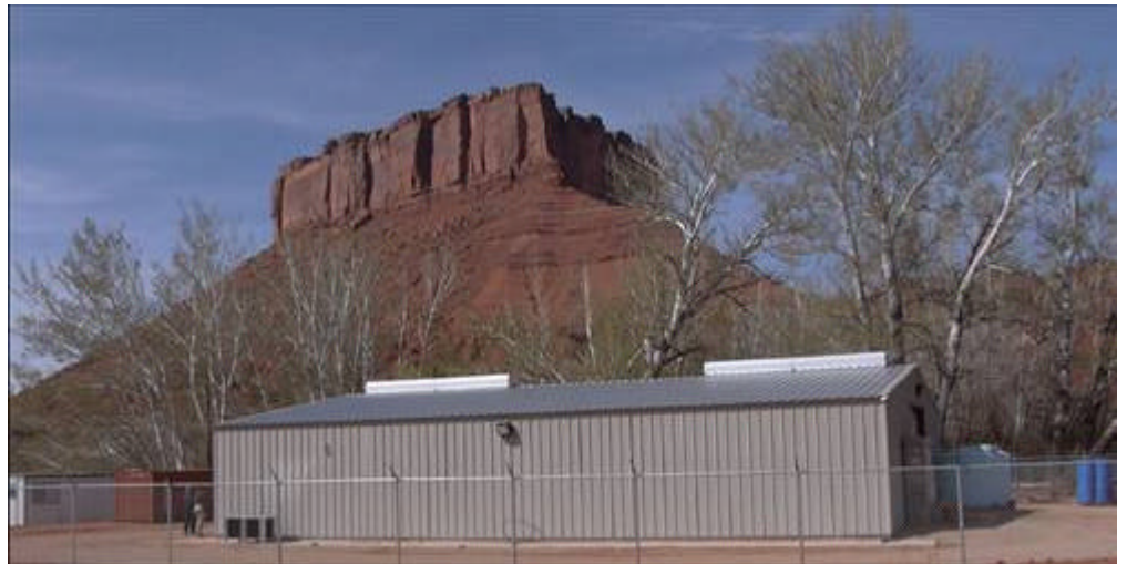
2 MWh VRB Energy Storage System at PacifiCorp
