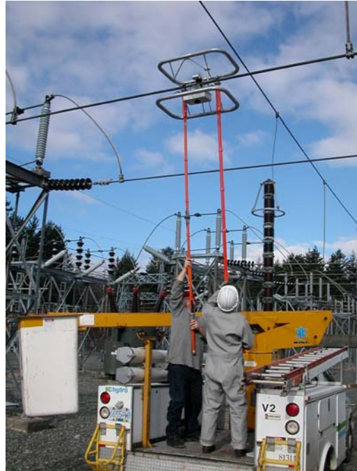
Figure 7. (above) Installing the HV Primary Sensor using hot sticks
