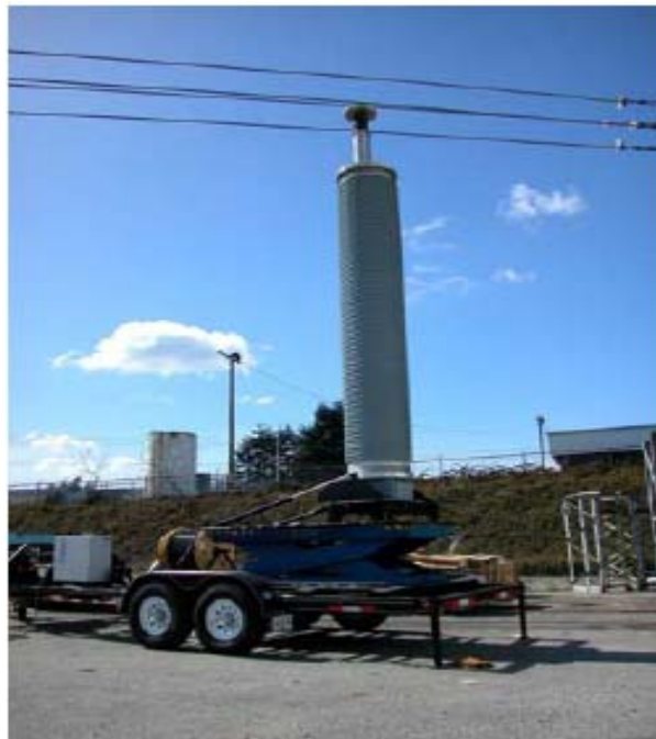
Fig 3. OVT Raised Into Contact With the Primary Bus
