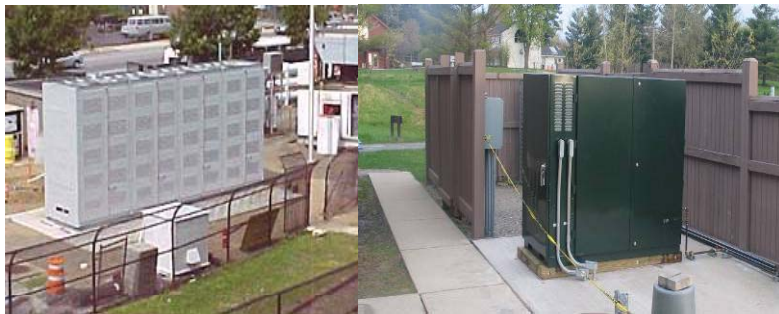
P94 Energy Storage
