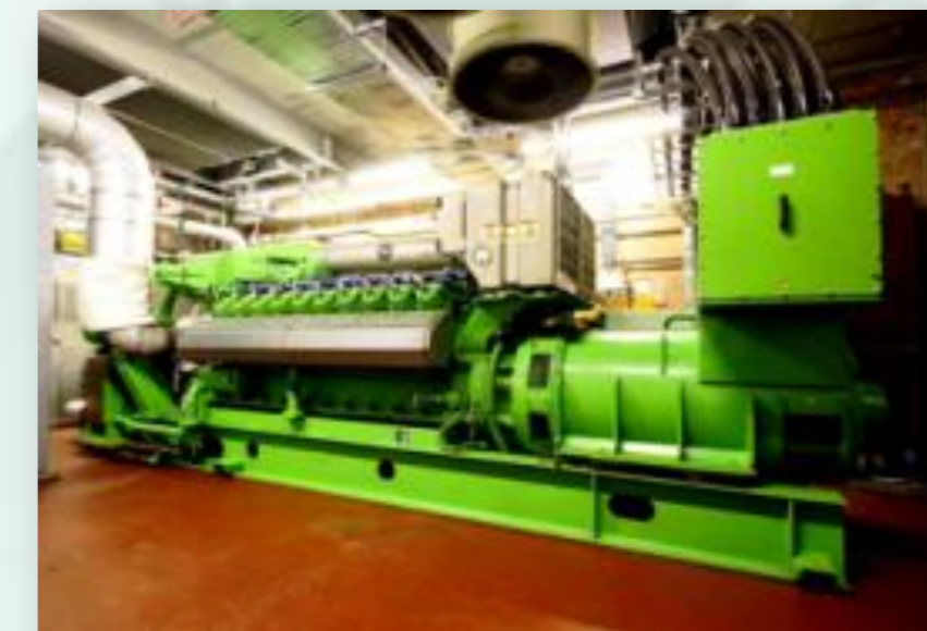
Combined Heat & Power
