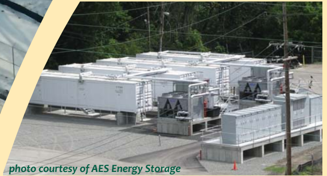
photo courtesy of AES Energy Storage
