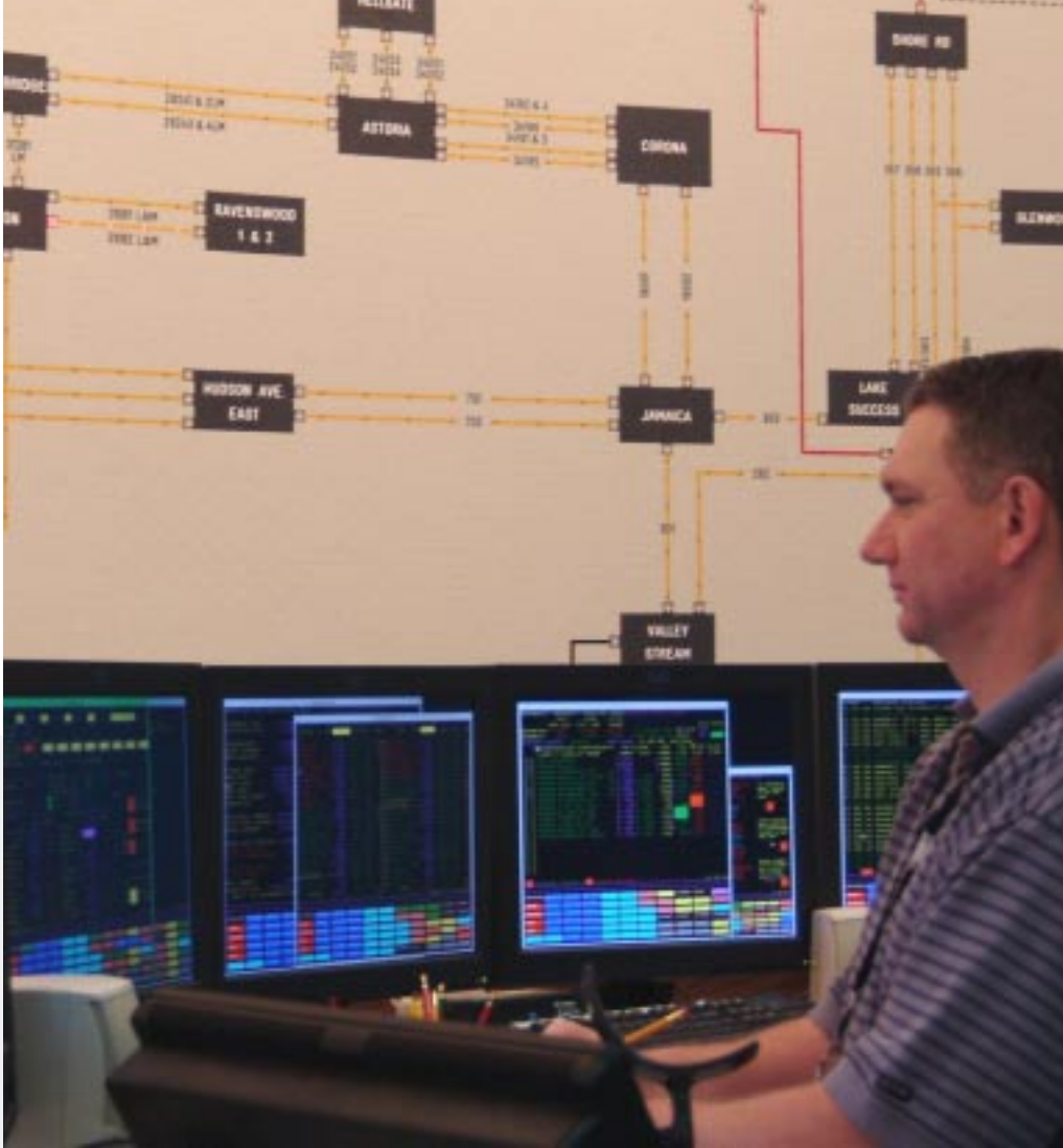
Patrick Shawver, Dispatcher, watches over the generation mix across New York State from his post in the NYISO control room.
