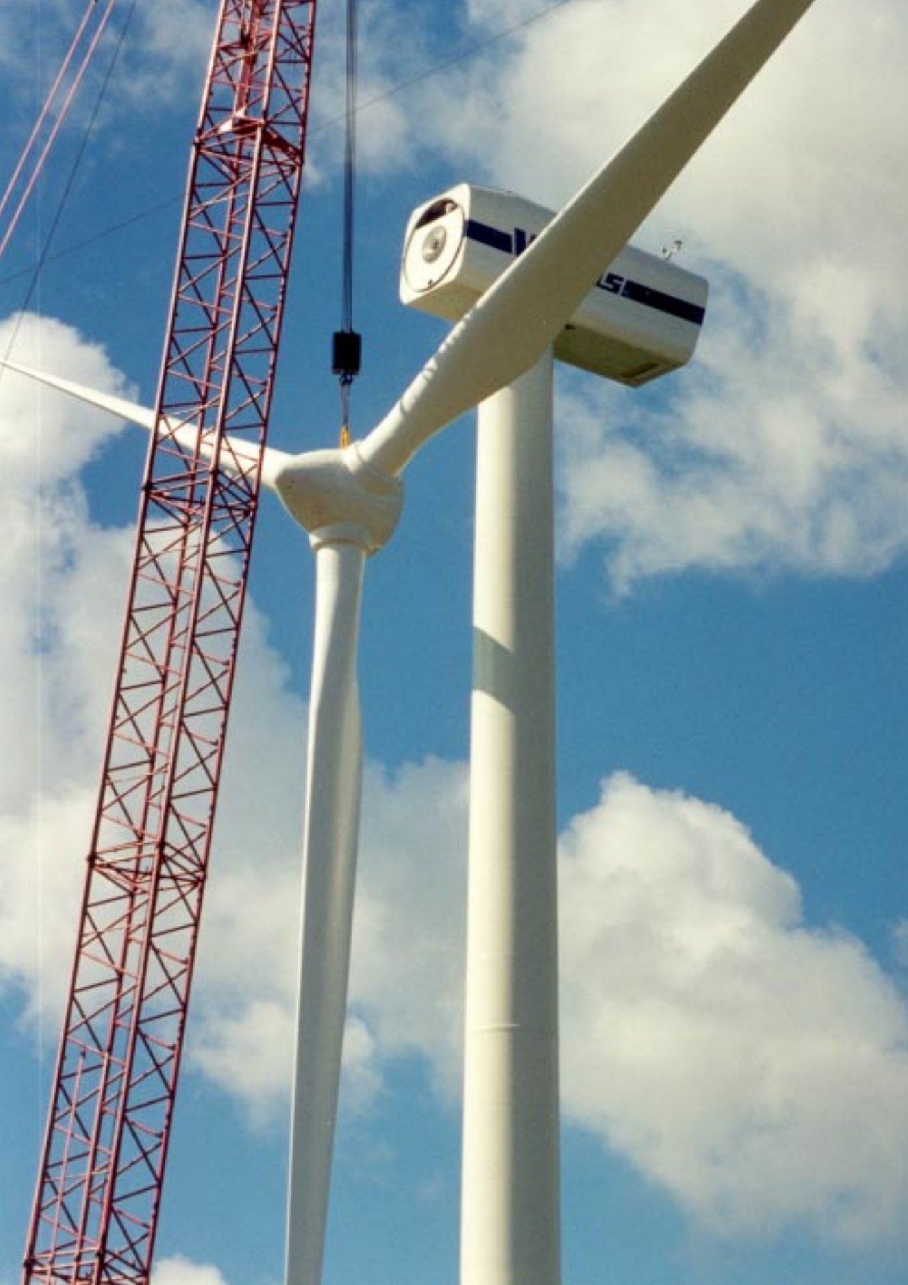
NEGT's Madison Windpower Project in Madison County is an example of the important role renewable energy sources play today and for the future. Madison's 7 wind turbines contain a total installed capacity of 9 megawatts.
