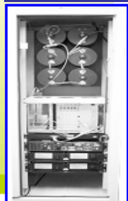
Examples of Base Station Equipment
